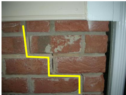
Step crack at top 4 courses
