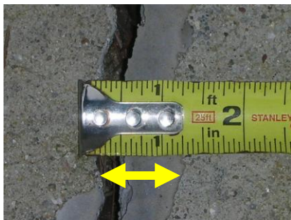
Driveway crack with failed sealant
