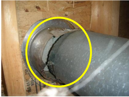
Down draft kitchen exhaust duct disconnected
