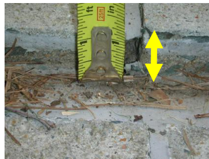
Driveway over an inch out of level
