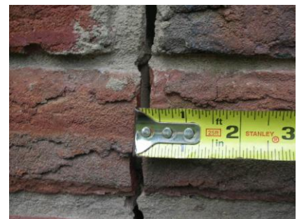
Close up photo of cracked brick
