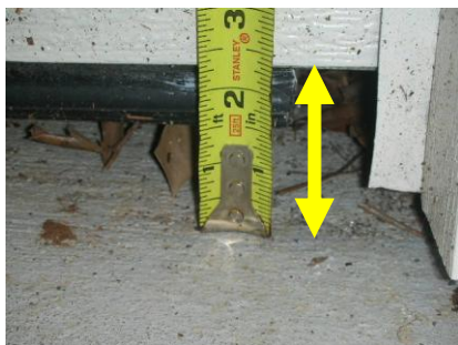
Gap at right side of garage door
