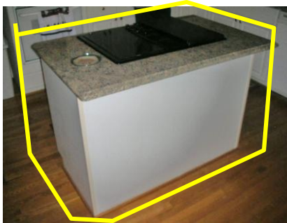
Kitchen island has no receptacle
