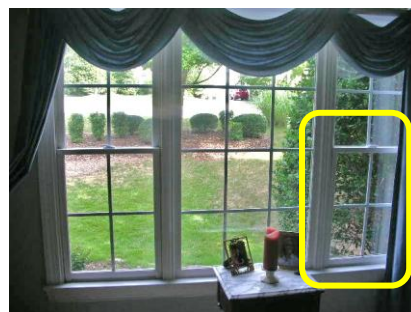
Lower sash not square in frame
