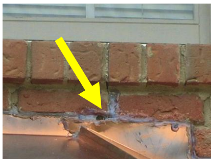
Dime sized hole over copper roof.
