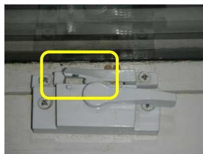
Broken window sash lock front bedroom
