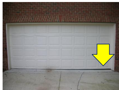
Wide angle photo of garage door gap
