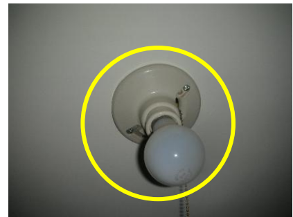
Closet light not enclosed
