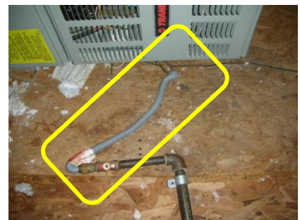
Missing sediment leg at attic furnace
