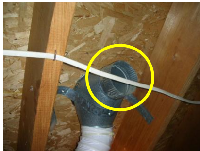
Metal Y missing hall bath duct
