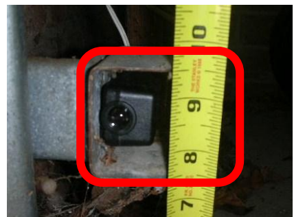
Garage motion sensor too high
