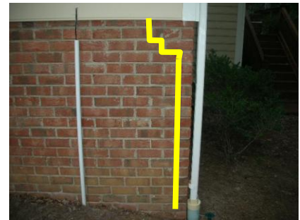
Vertical crack at left rear corner
