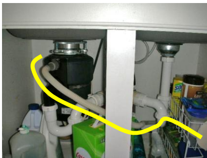
Dishwasher drain missing high loop
