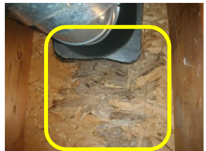
Water stains on roof sheathing
