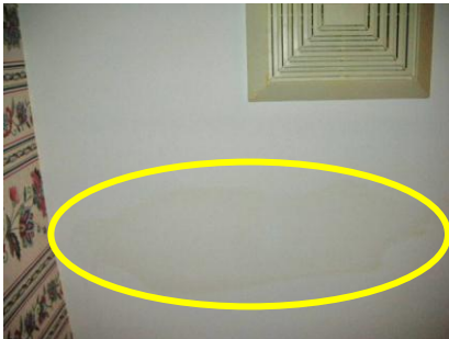
Water stain 1 st floor bath ceiling
