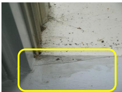
Water stained window sill living room
