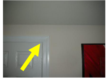
Music room closet door binds
