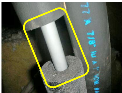
Polybutylene plumbing at water heater
