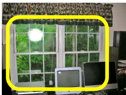
Double pane seals failed
