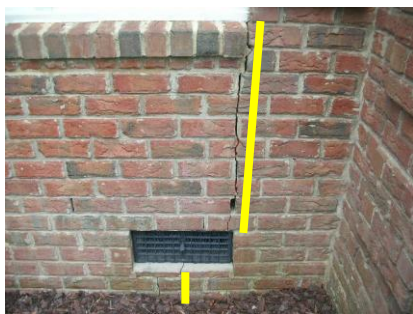
Crack in brick under living room window
