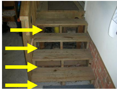
Oversized opening in garage stair
