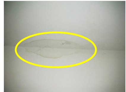
Water stain master closet ceiling
