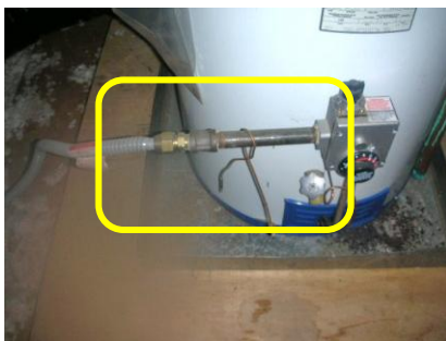
Missing sediment leg at water heater
